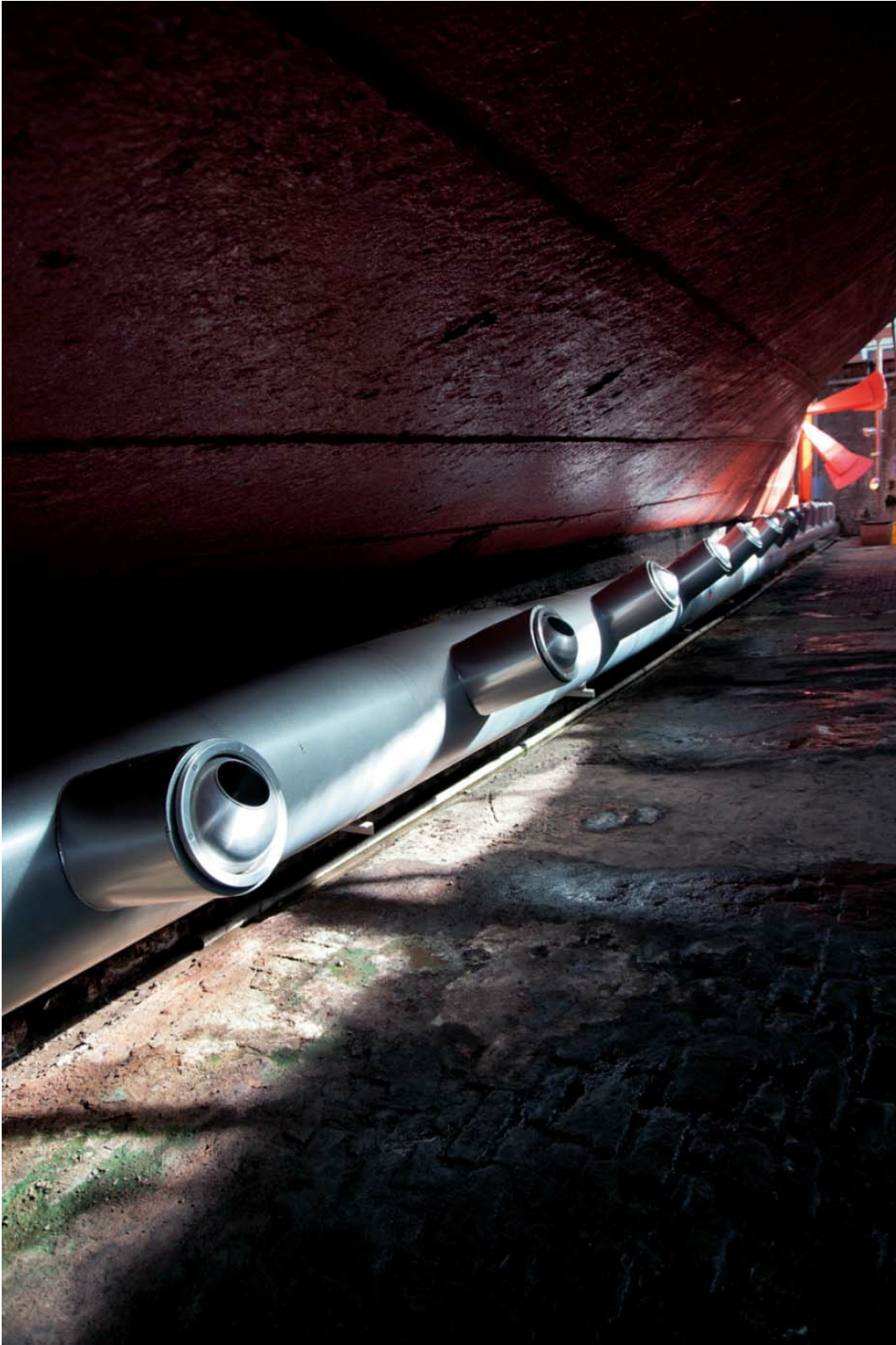
A view of the ducts for the lower hull's external dry air supply, arranged either side of the keel to create an upward flow of air, blanketing the iron plates and inhibiting the chloride corrosion that has proved so destructive.
