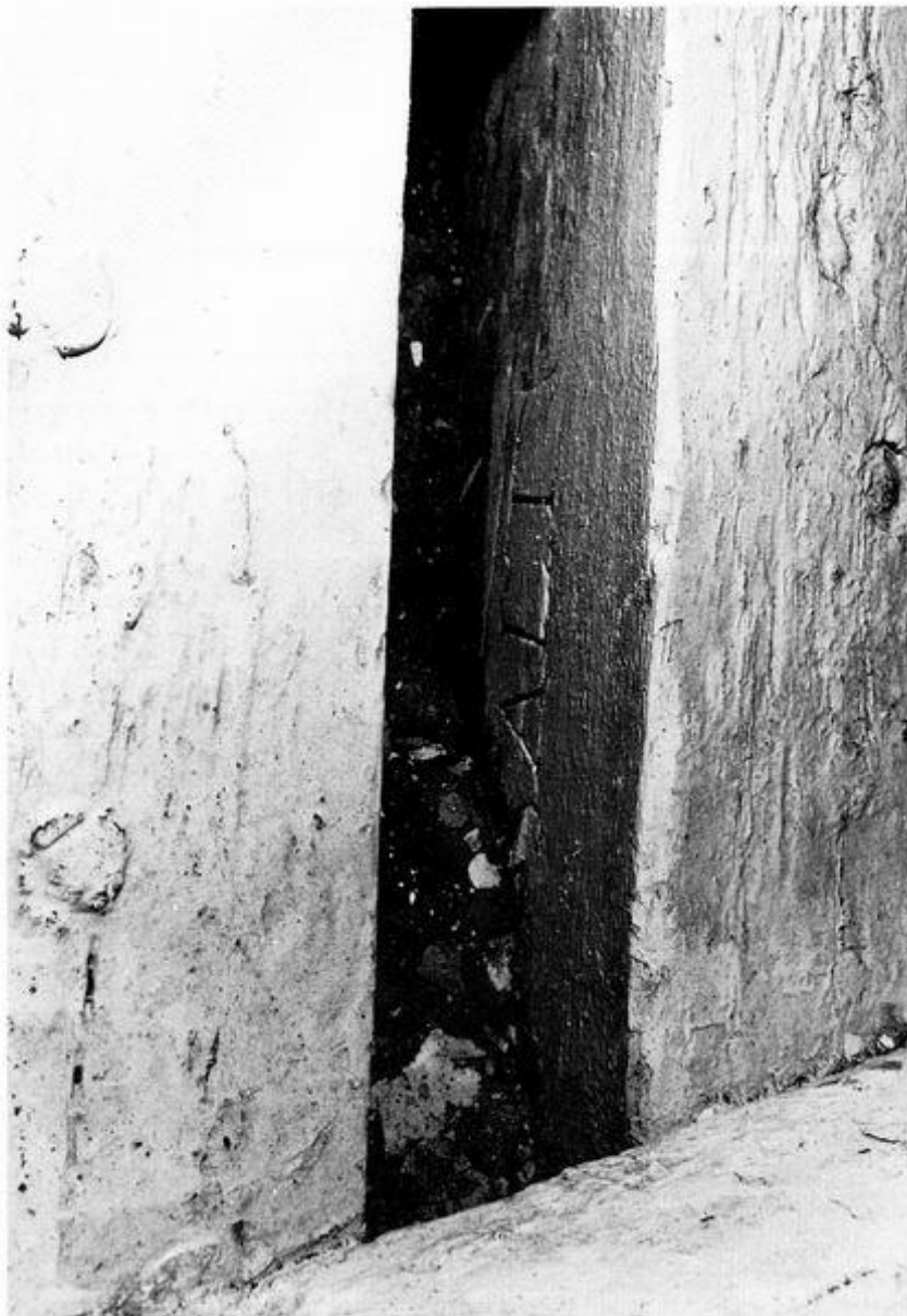
Unicorn. Close-up of the spacing between the timbers, starboard side, forward, showing the 'race' mark 'SALT', which indicated that this timber had been pickled in brine prior to its use. This practice was introduced by Seppings to prevent the premature rotting of frames.
