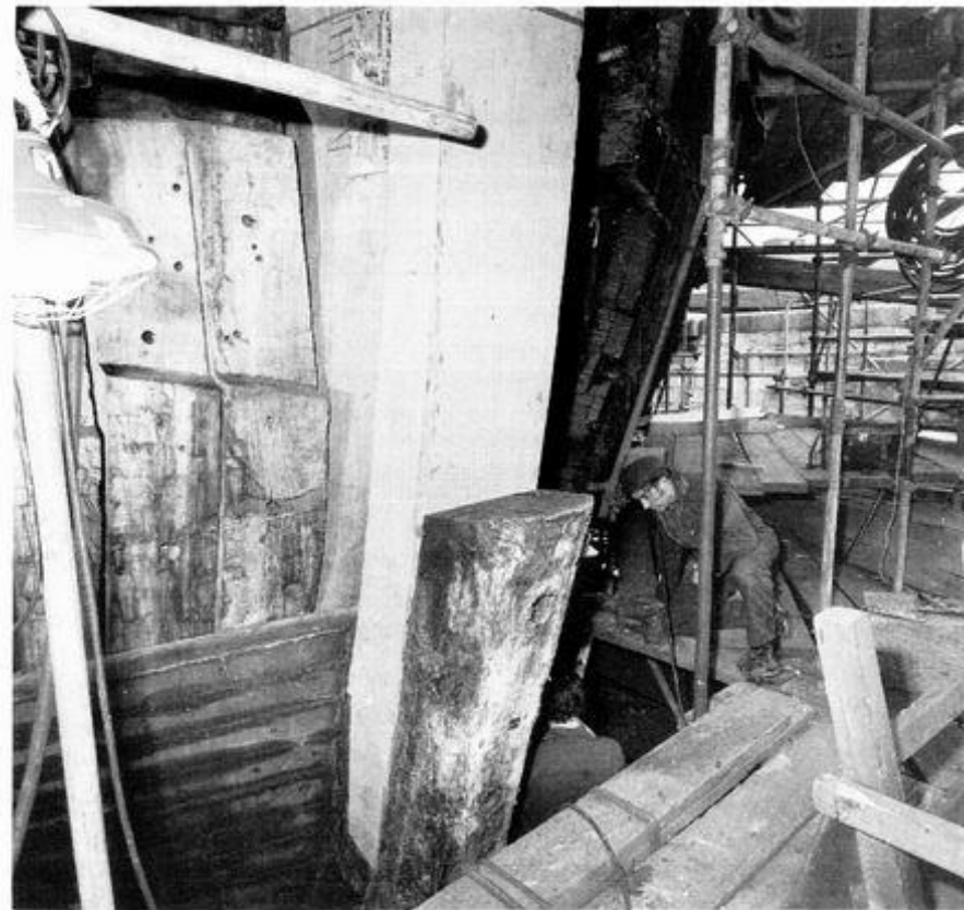
Victory. Starboard side of stempost. This view shows a new section of the stem being fitted to the foreside of the apron. The house pieces, the rabbet, the hood ends of the planking and the upper part of the gripe are also discernible. Note the diminishing strakes at the top right corner of the photograph.
