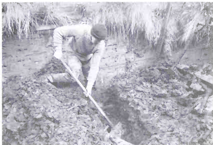
Fig 273. The author digging a trench through the mud and debris on the inside of the Millom Castle in order to take offsets.
